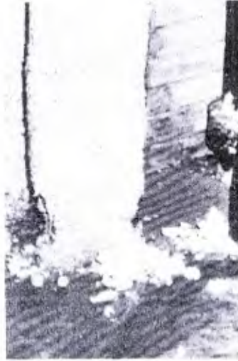
ACM which physical condition and normally deteriorate insulation
