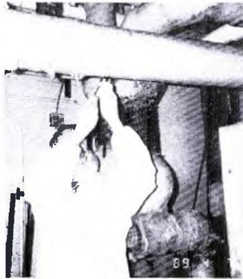
A properly trained and protected building inspector collecting a bulk sample of suspected asbestos-containing thermal system insulation.
